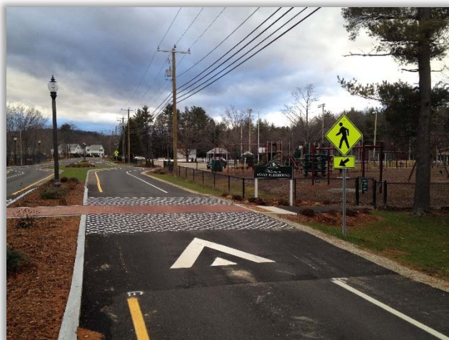
Peterborough, NH – Union Street Roadway Reconstruction, Pedestrian Facilities, Stormwater, Sewer Replacement, Lighting
